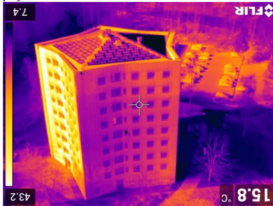
Figure 6: Thermographic imaging of Stackens BIPV facades and roof from a drone mounted IR camera.
